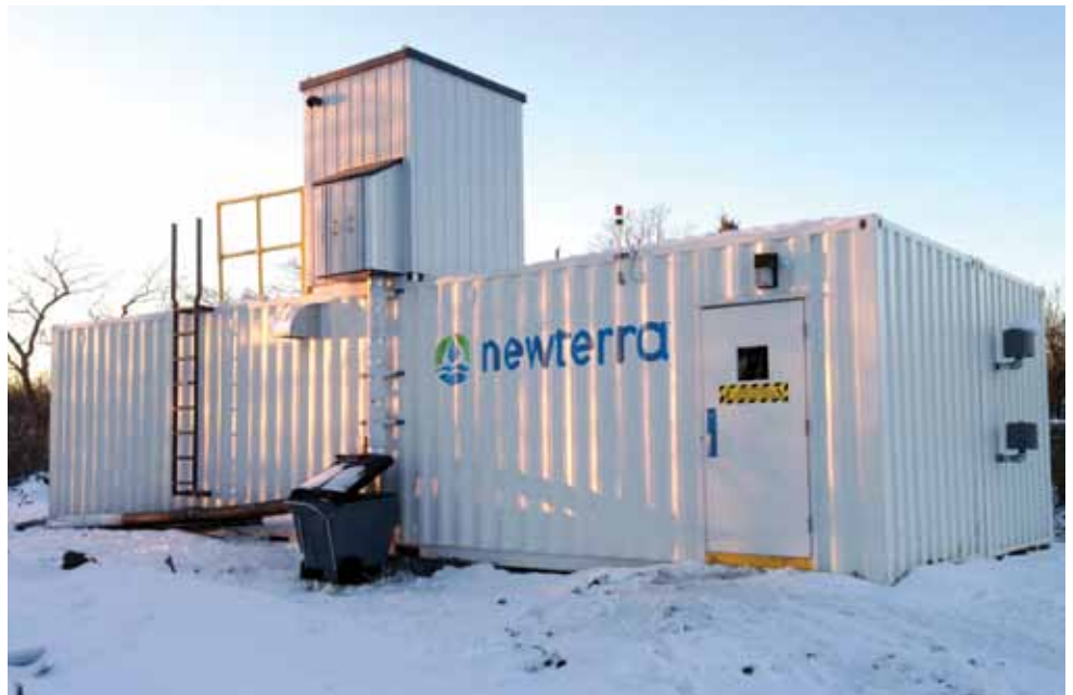
Decentralized systems offer advanced treatment technologies in a very compact footprint. This modular MBR system at an Ontario RV park treats 83 m3 of sewage per day yet requires only 16' x 40' of space.
