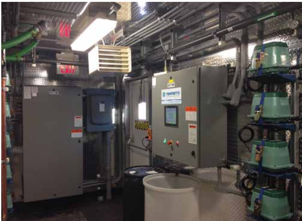
With full automation and remote system monitoring and control, modern decentralized systems operate with minimal maintenance or operator involvement.
